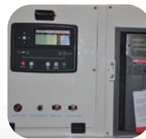
Control Panel & MCB
